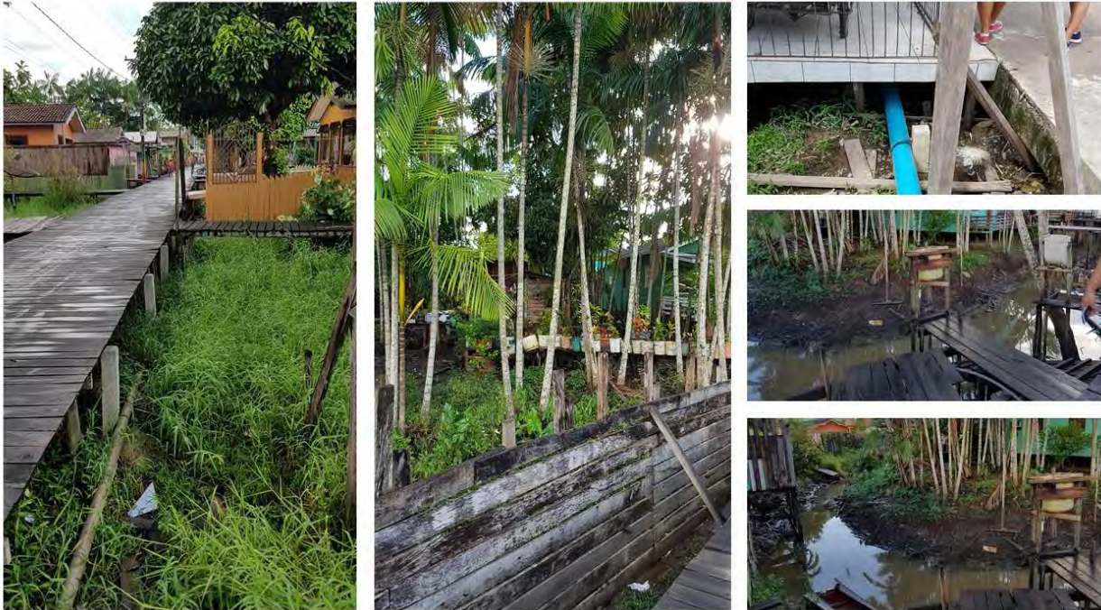
Figure 34.2 Infrastructure deficit in the city of Afuá, Pará, Brazil (Source: Laboratório de Estudo das Cidades Collection/UNIVAP).
